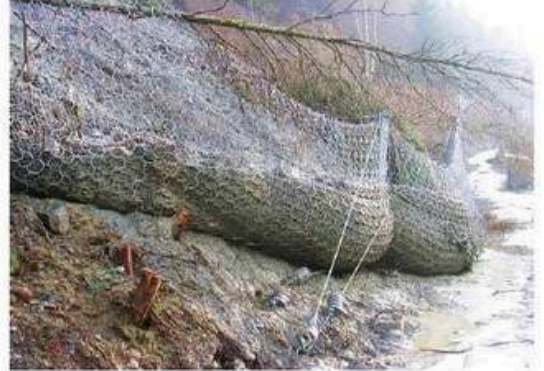
Debris Flow Barriers
